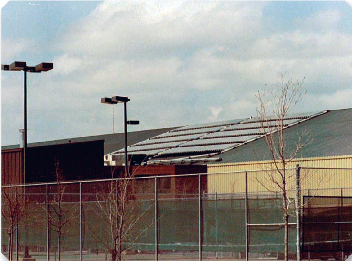
Solar heating system at the Ottawa Athletic Club installed by Davis Engineering.
